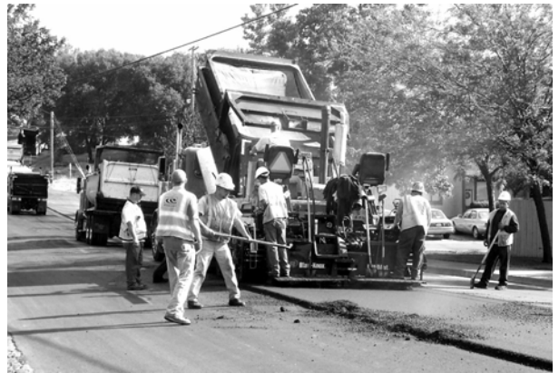
Central Valley Engineering & Asphalt crews paving Old Highway 53 between Olympic Drive and Lakeshore.
